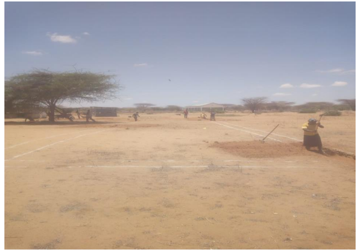
Construction of dining hall begins on 31 st march 2019 at NEYD Orphanage Centre
